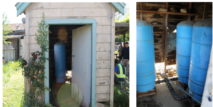
Figure 3 - Pump, Pumphouse, three storage tanks from the assessment trip. Located in the backyard of 742 Middlefield Rd.
